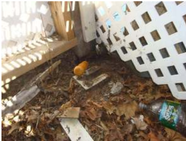
5. ROTTED AND MISALIGNED POST
