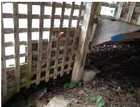
○ Post off of pier condition.
