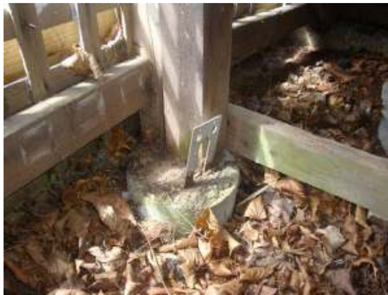
6. MISALIGNED POST AND CONCRETE POST
