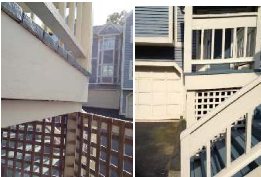
○ Out of alignment corner post condition.
