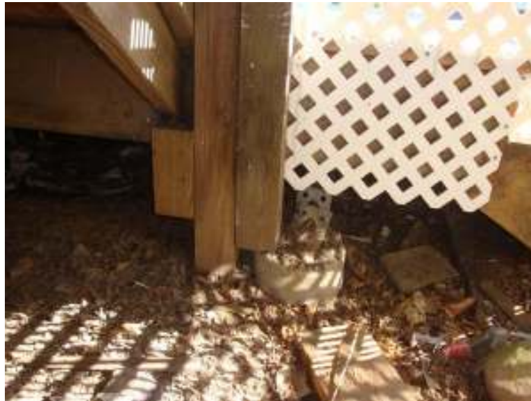
7. MISALIGNED POST AND CONCRETE POST
