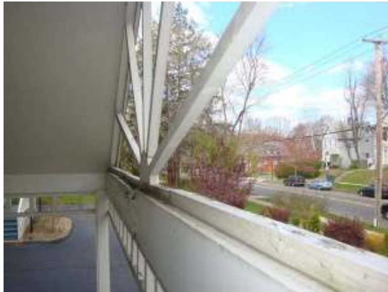
9. WATER DAMAGED GABLE TIE BEAM
